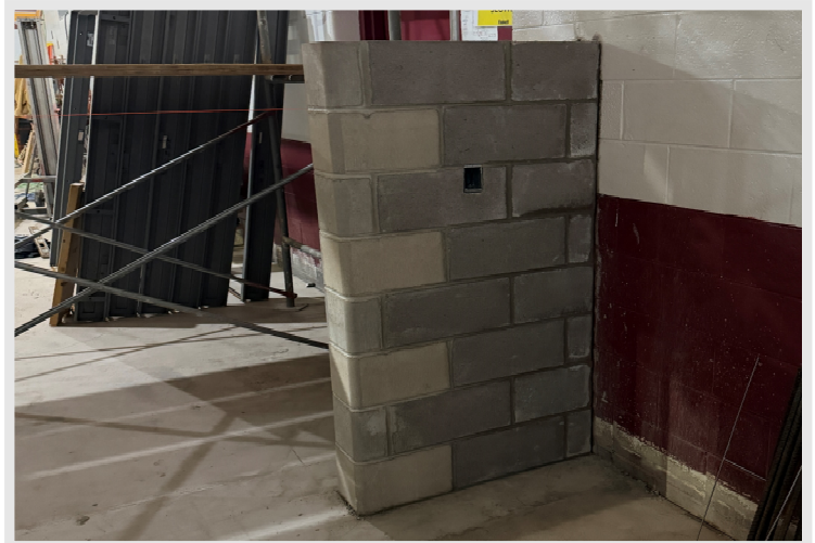
The masons have begun working on the opening between the new band room and band storage.
