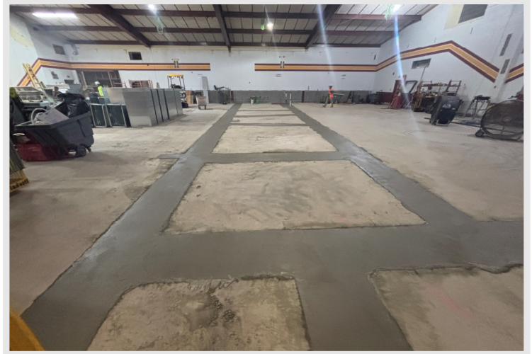
The thickened concrete footings have been poured back to get ready for masonry walls.
