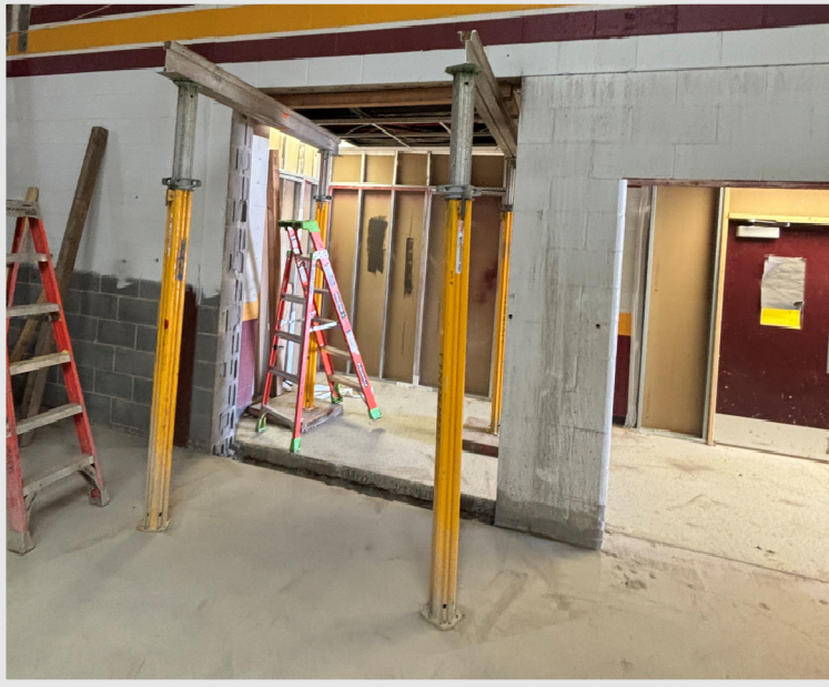
The new door openings have been cut and have been prepped for new overhead lintels
