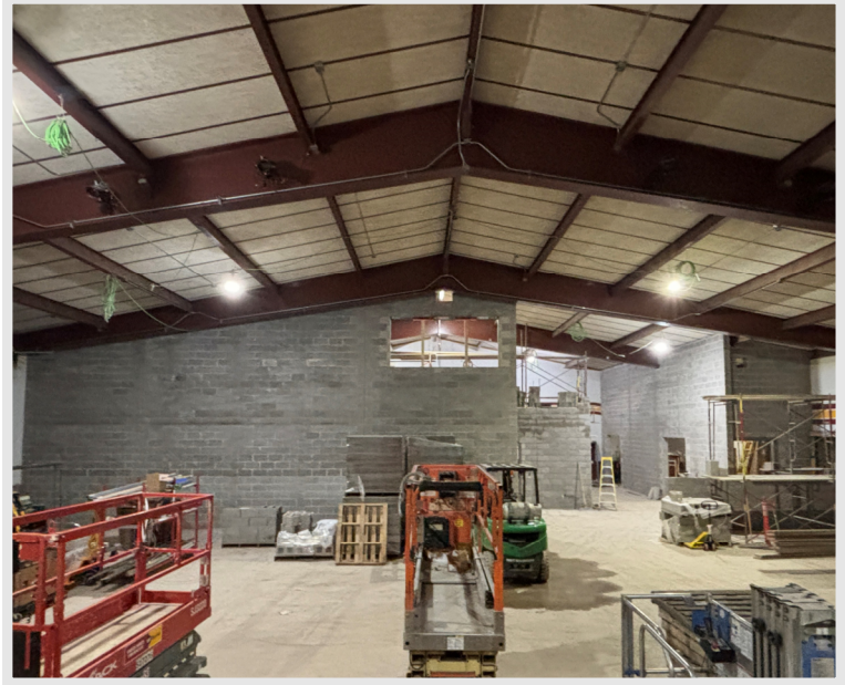
A view from the stage looking back towards the new band room walls.
