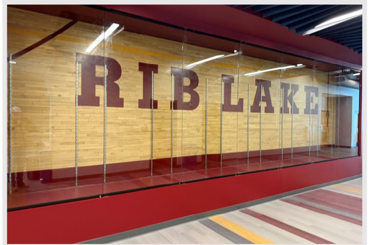
The Display Case work is near completion with the installation of the glass doors.
