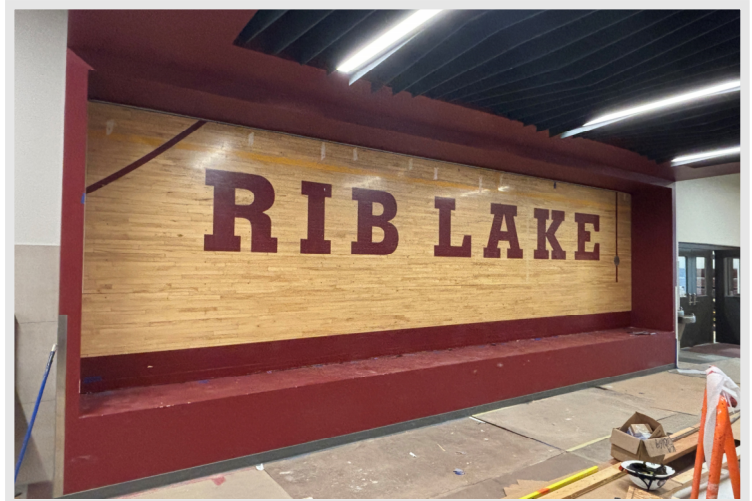
The existing gym floor cutout has been set into place as the background of the addition trophy case.
