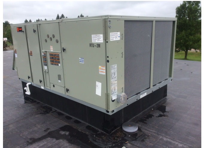
New Roof top HVAC unit at the Middle School
