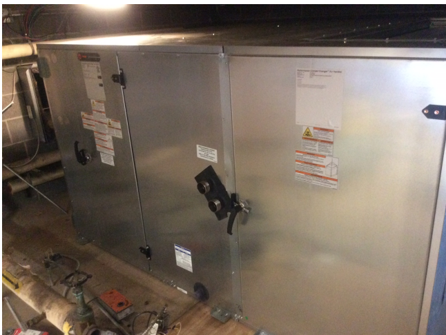
A new air handling unit above the stage is currently being completed.
