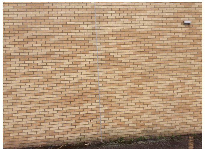
Exterior caulking has failed but has been replaced and properly installed on all three schools.
