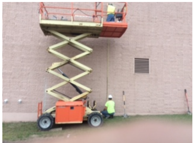
An overhead door is being installed to accommodate the new biomass boiler and related equipment.
