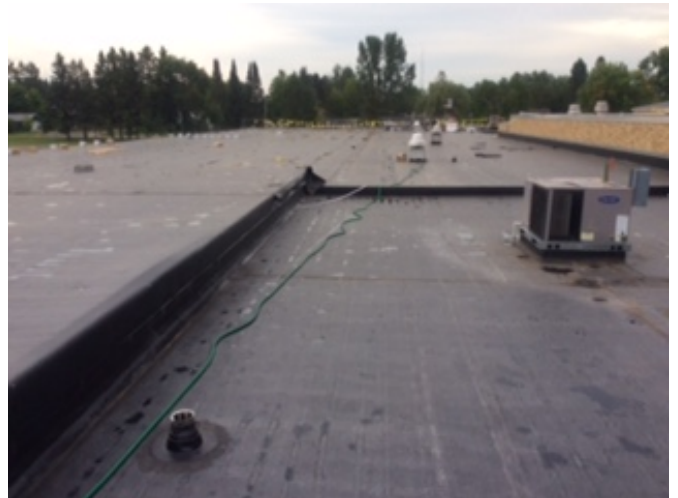
New fully adhered membrane roofing is nearly complete in selected areas at the High School.
