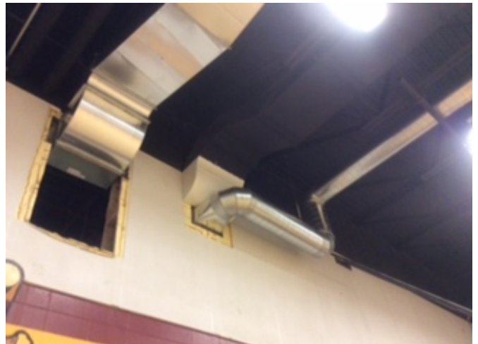
Sheet metal air distribution ducts are nearly complete at the Middle School
