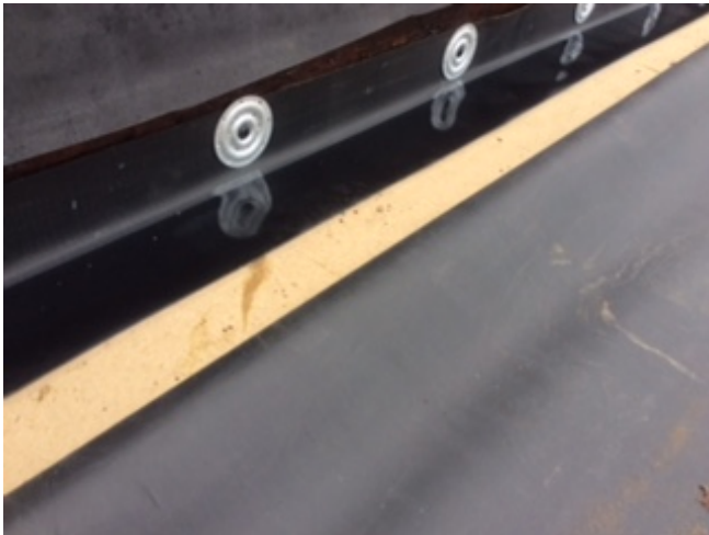
Improved roofing details. Architectural sheet metal will be installed during the month of August.
