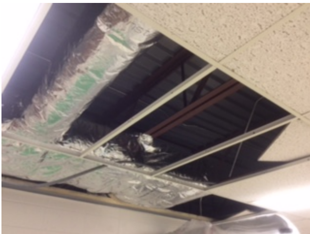
The sheet metal HVAC ductwork is nearly complete and is currently being insulated in the Middle School.
