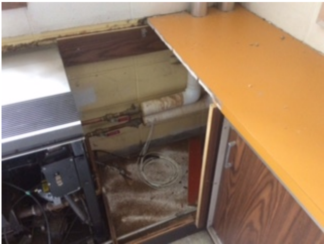
The removal of some unit ventilators has been challenging but surrounding materials will be replaced following the installation of new equipment.
