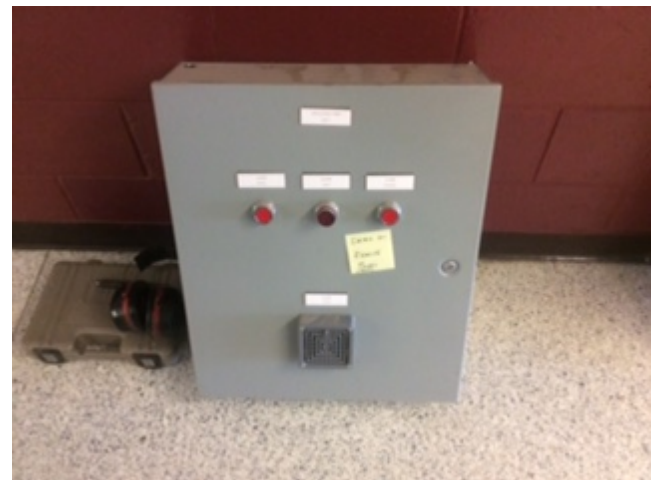
An old removed control panel. Electrical and equipment controls will be upgraded.
