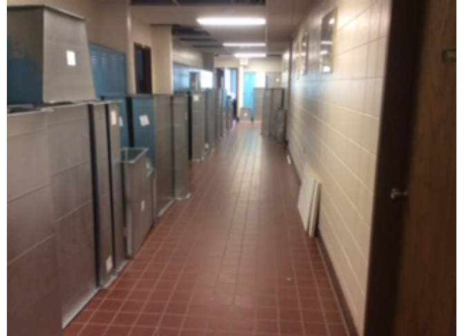
New ductwork in the Middle School will be installed during the month of July.
