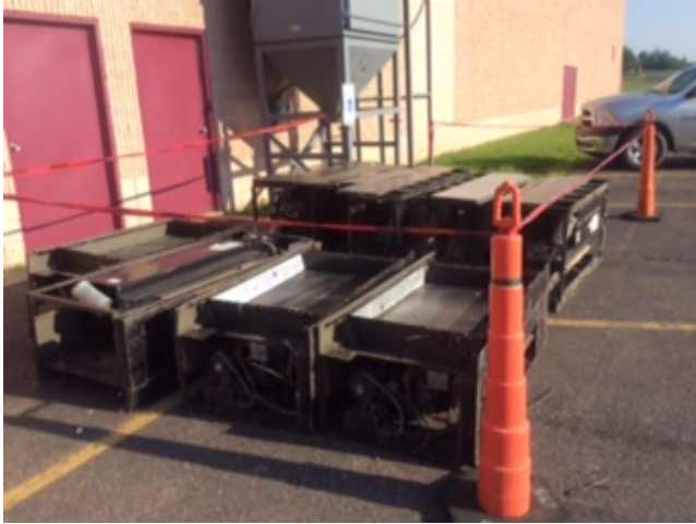
Most of the classroom Unit Ventilators have been removed in the Middle School.
