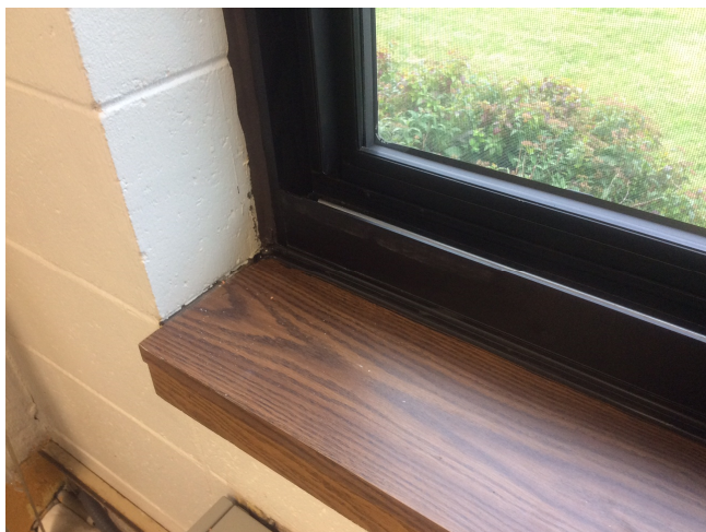
A typical sill condition of the new anodized aluminum windows in the Middle School.
